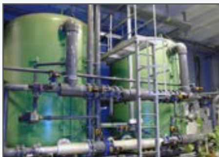
Environmental protection equipment
